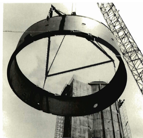
Tower of power, the Holifield Heavy Ion Research Facility, here under construction in 1977, would become the world’s most powerful heavy-ion accelerator.
